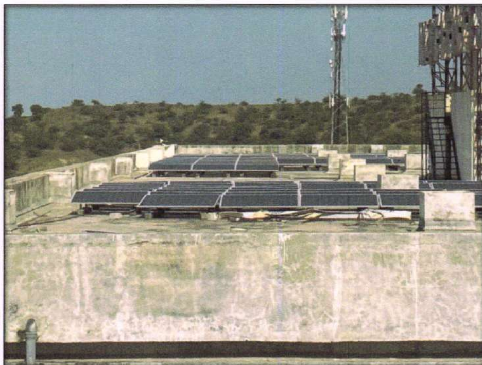
Photograph of Solar PV Plant:
