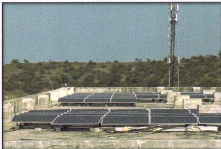
Photograph of Solar PV Plant:
