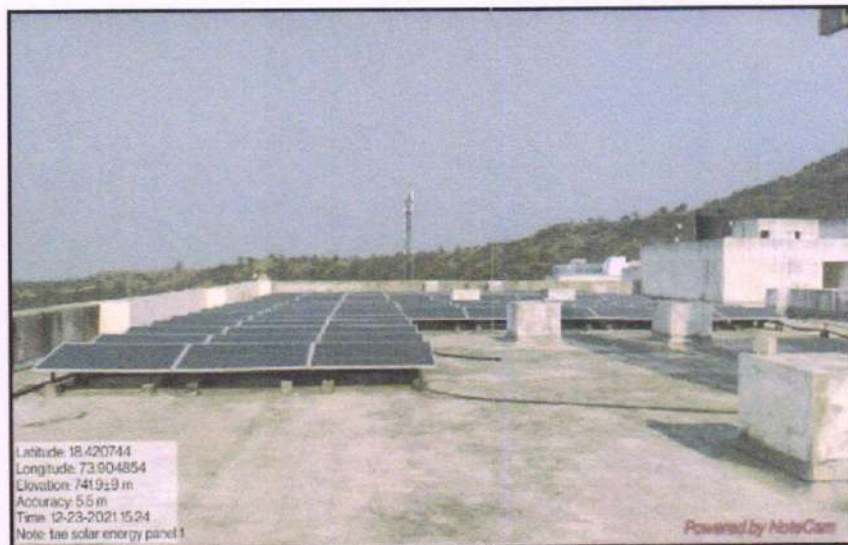
Photograph of Roof Top Solar PV Plant:
